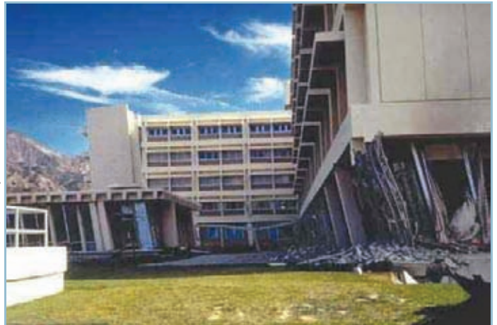
In 1971, a 6.7 earthquake severely damaged the Olive View Psychiatric Hospital in San Fernando, California
