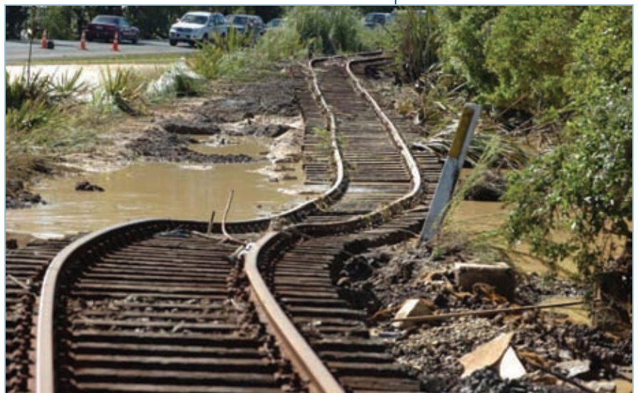
Its not just earthquakes that buckle railway lines
