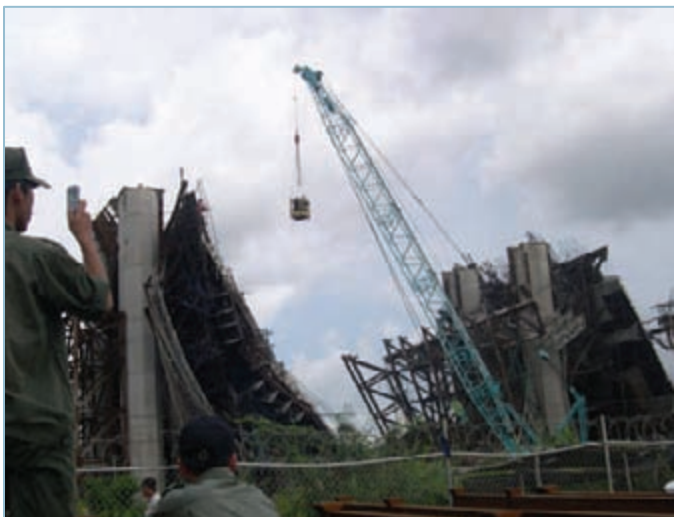
The collapsed section of the bridge
