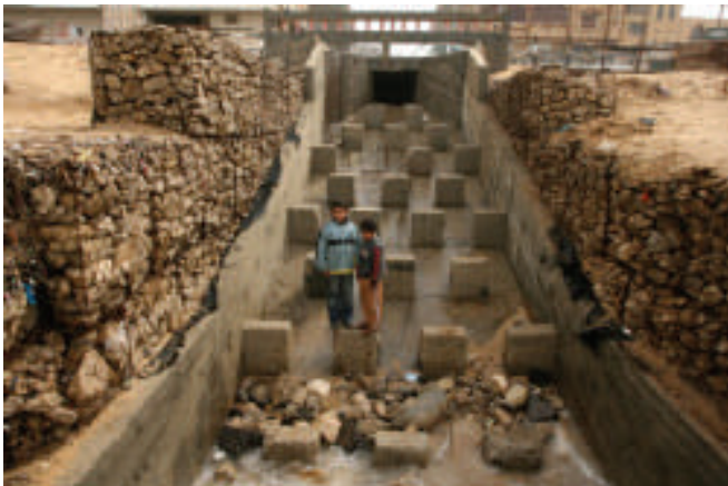
A point near the Beach refugee camp where sewage, either partially treated or not at all, runs into the sea
